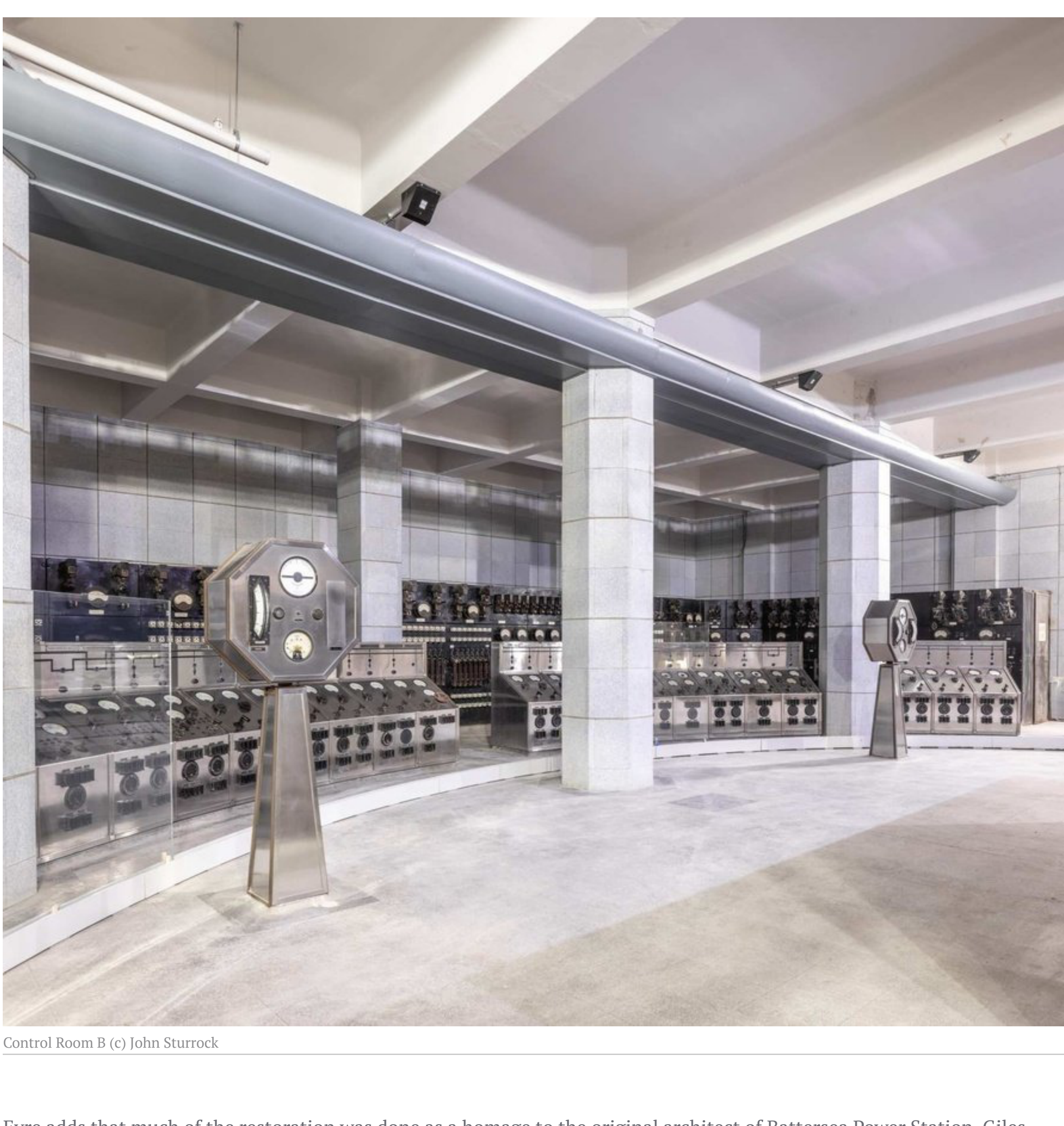
Control Room B (c) John Sturrock
